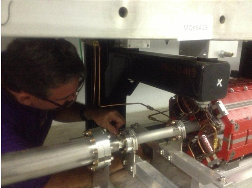
West Arc LCW connections to magnets
