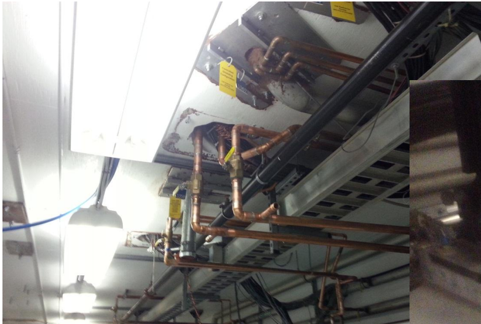
LCW installation in 1S
